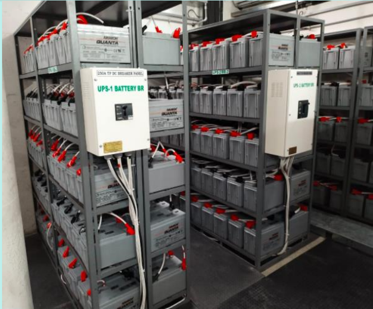
New UPS system
