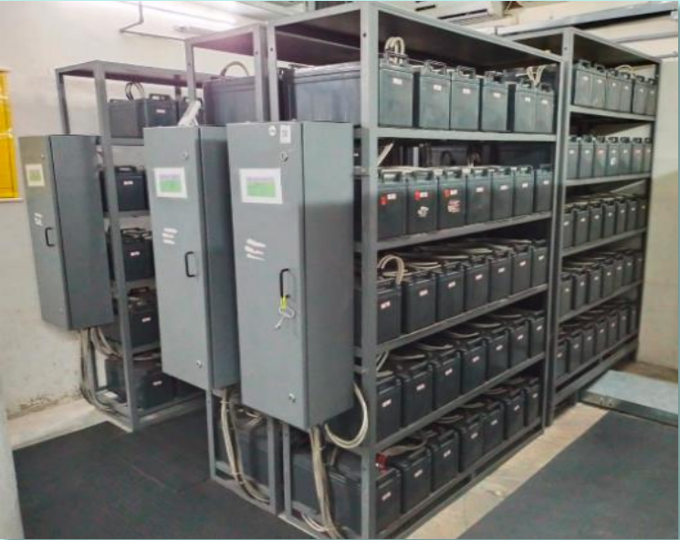
Old UPS system
